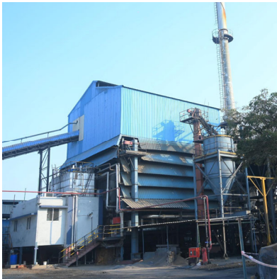
16 TPH Solid Fuel Boiler
